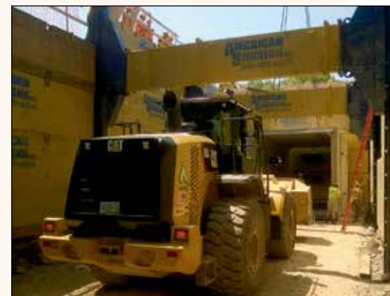
Inside shoring, a CAT 966 Loader passes beneath rolling strut to push culvert sections together.
