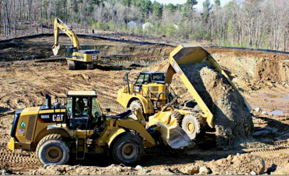
A CAT 966 Loader waits to spread excavated material deposited by a CAT 735C Off-Highway Truck as a CAT excavator works in background.
