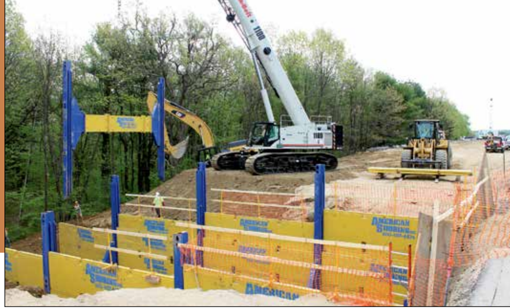
A Link-Belt TCC1100 Crane helps assemble components for American Shoring's double wall slide-rail system being used to support trench for 12-foot by 12-foot box culvert pedestrian underpass.
